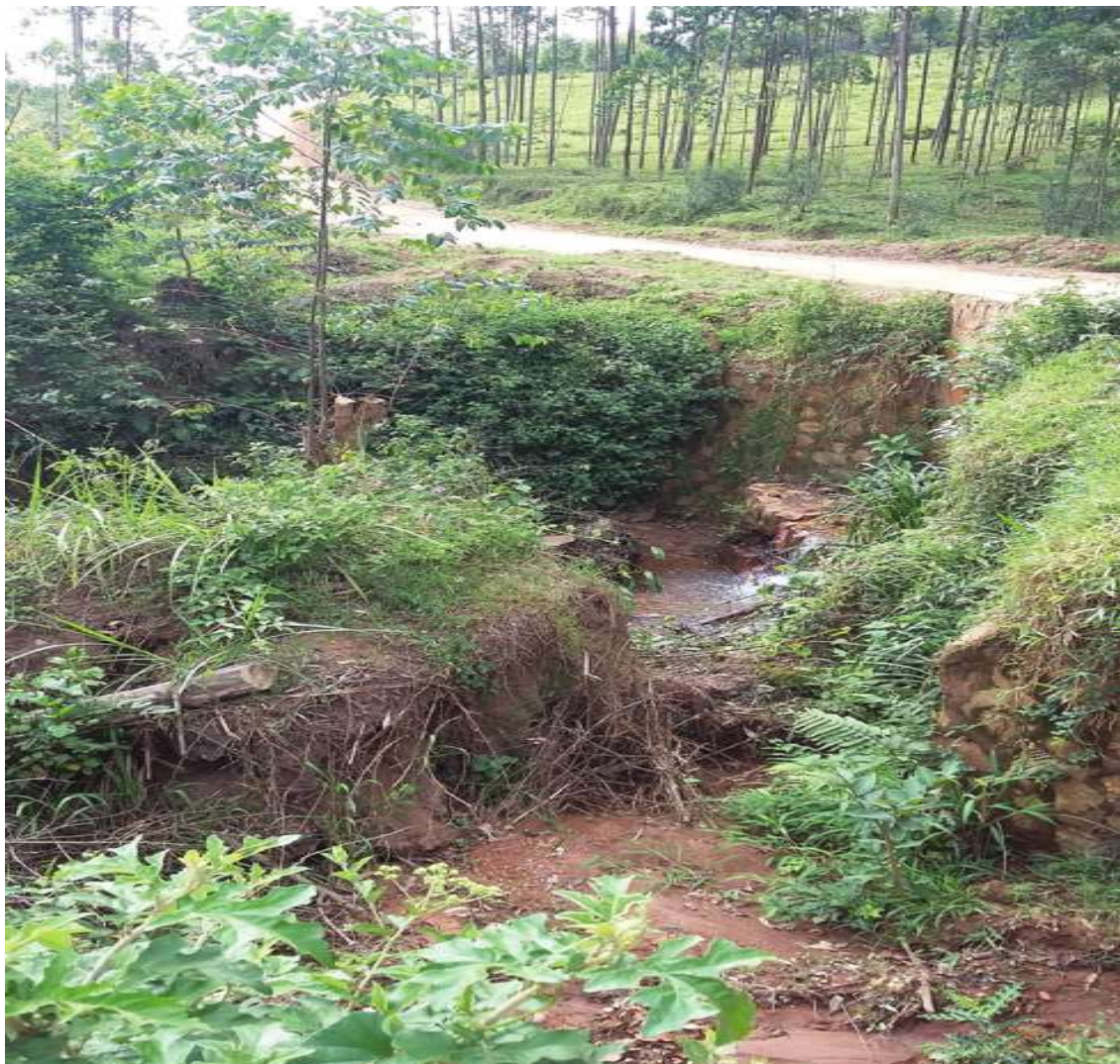
Plate 3: Flooding spot at Kanyeganyege culvert crossing, Buhunga Sub-county
